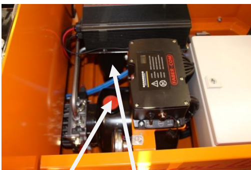
Hydraulic tank and pressure filter
