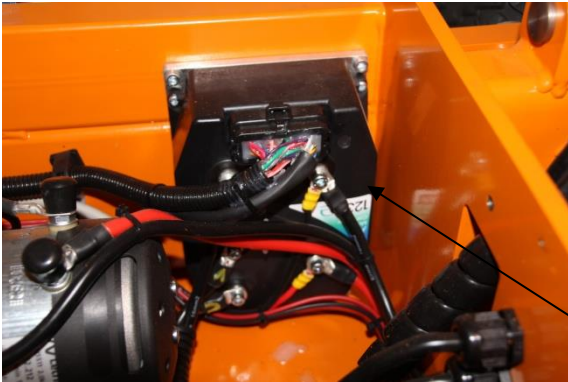
Motor control unit
